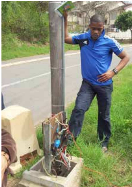
Example of an illegal electricity connection in South Africa. From [11]
