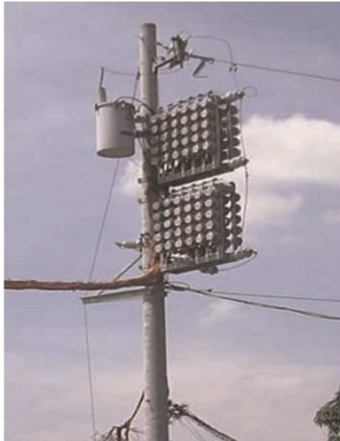
An elevated metering cluster, used to electrify informal settlements with less risk of tampering and illegality. Source: Meralco, "Delivering electricity to vulnerable communities", Asian Development Bank Asia Clean Energy Forum, June 19th 2009.
